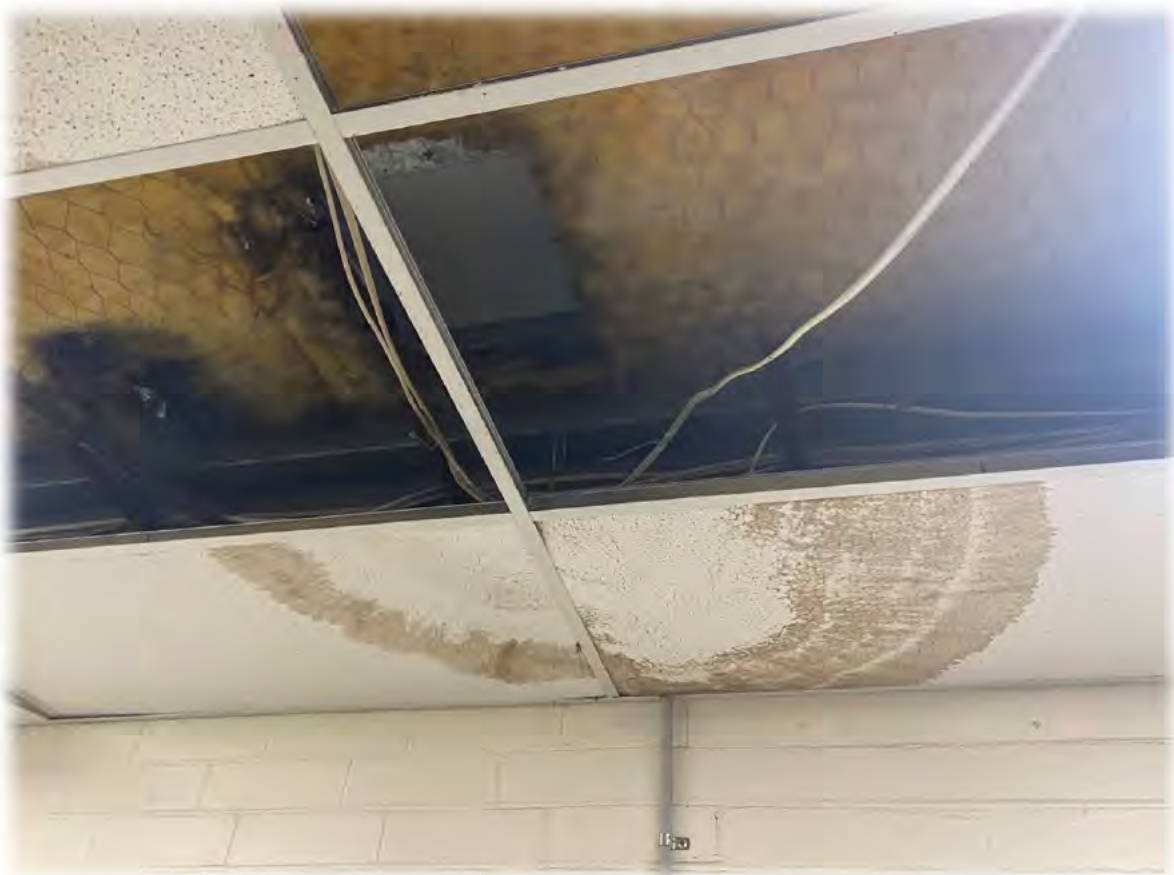
Figure 20: Damaged ceiling due to roof leak
