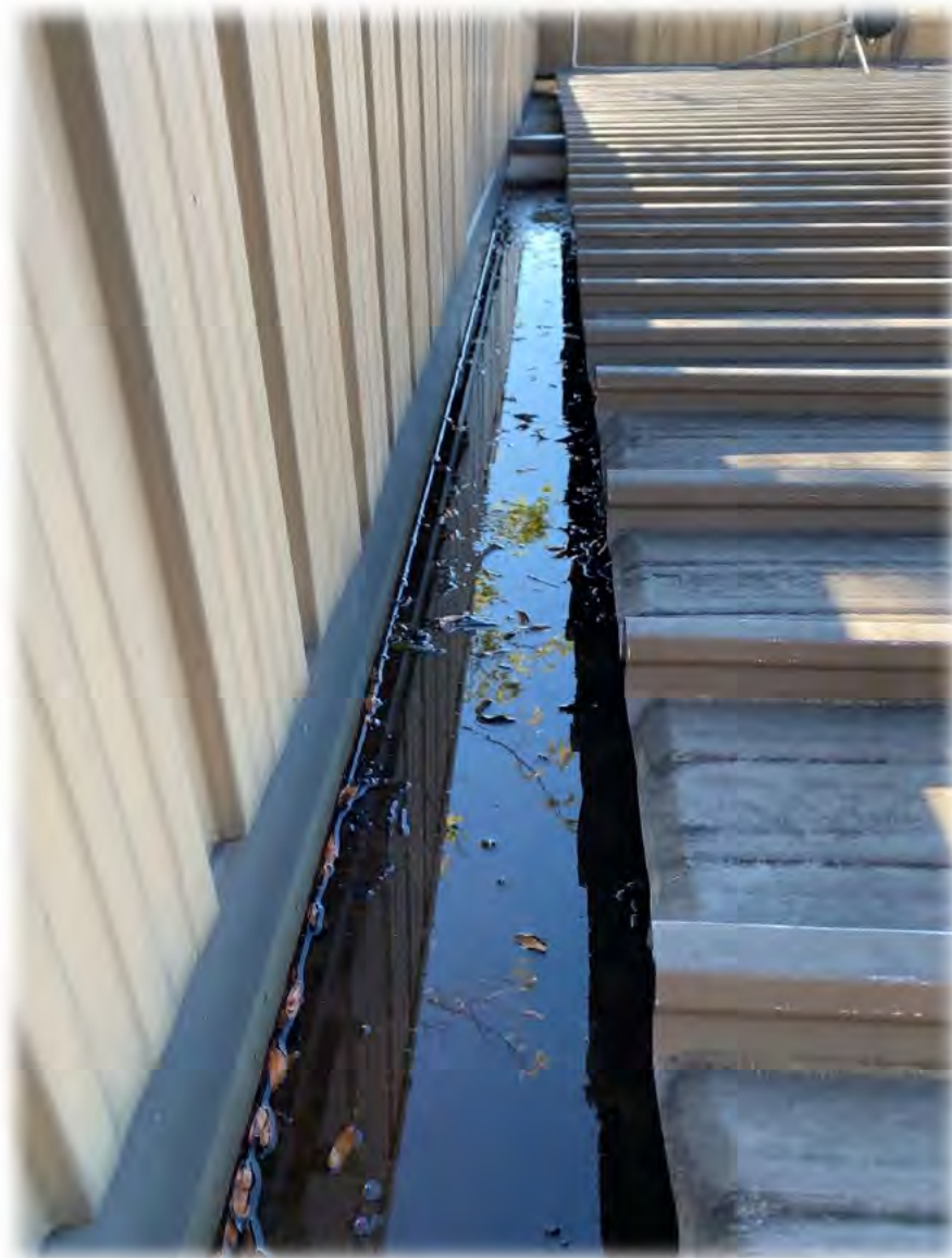
Figure 24: Flooded box gutter
