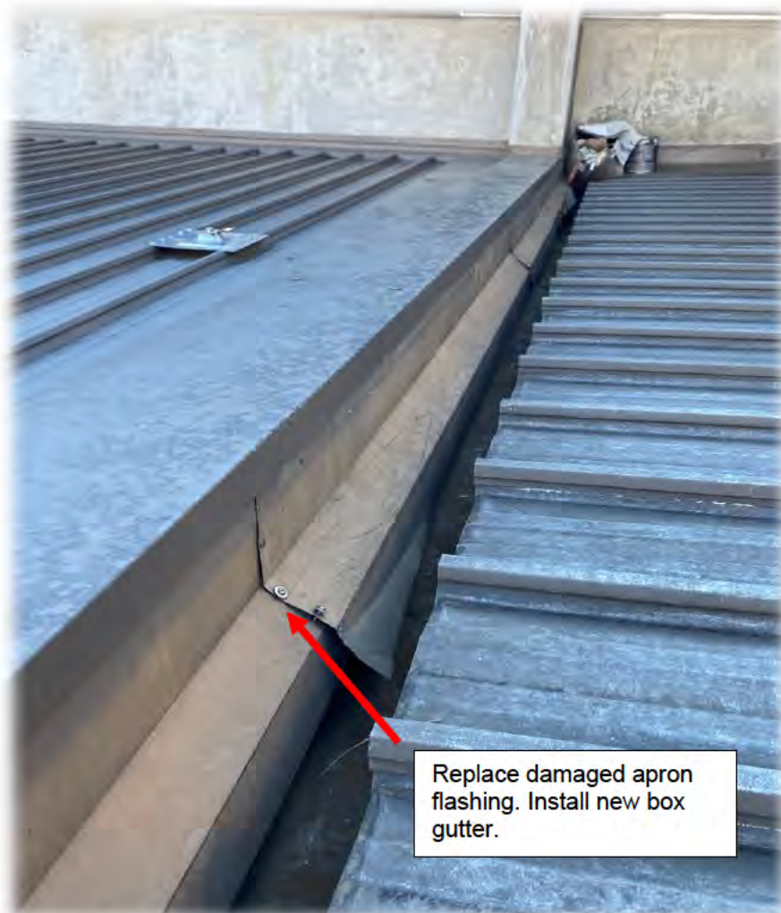
Figure 4: Damaged apron flashing
