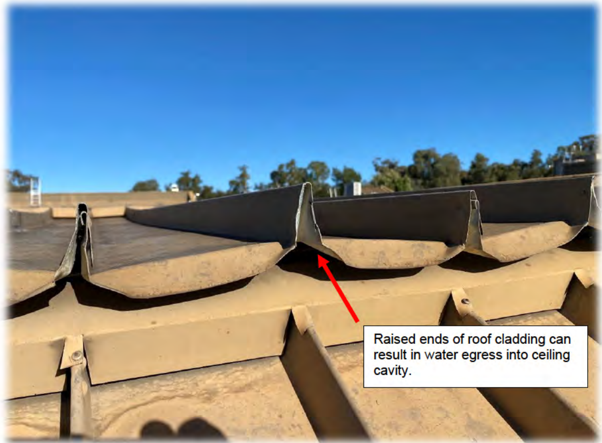
Figure 27: Lifted ends of roof cladding
