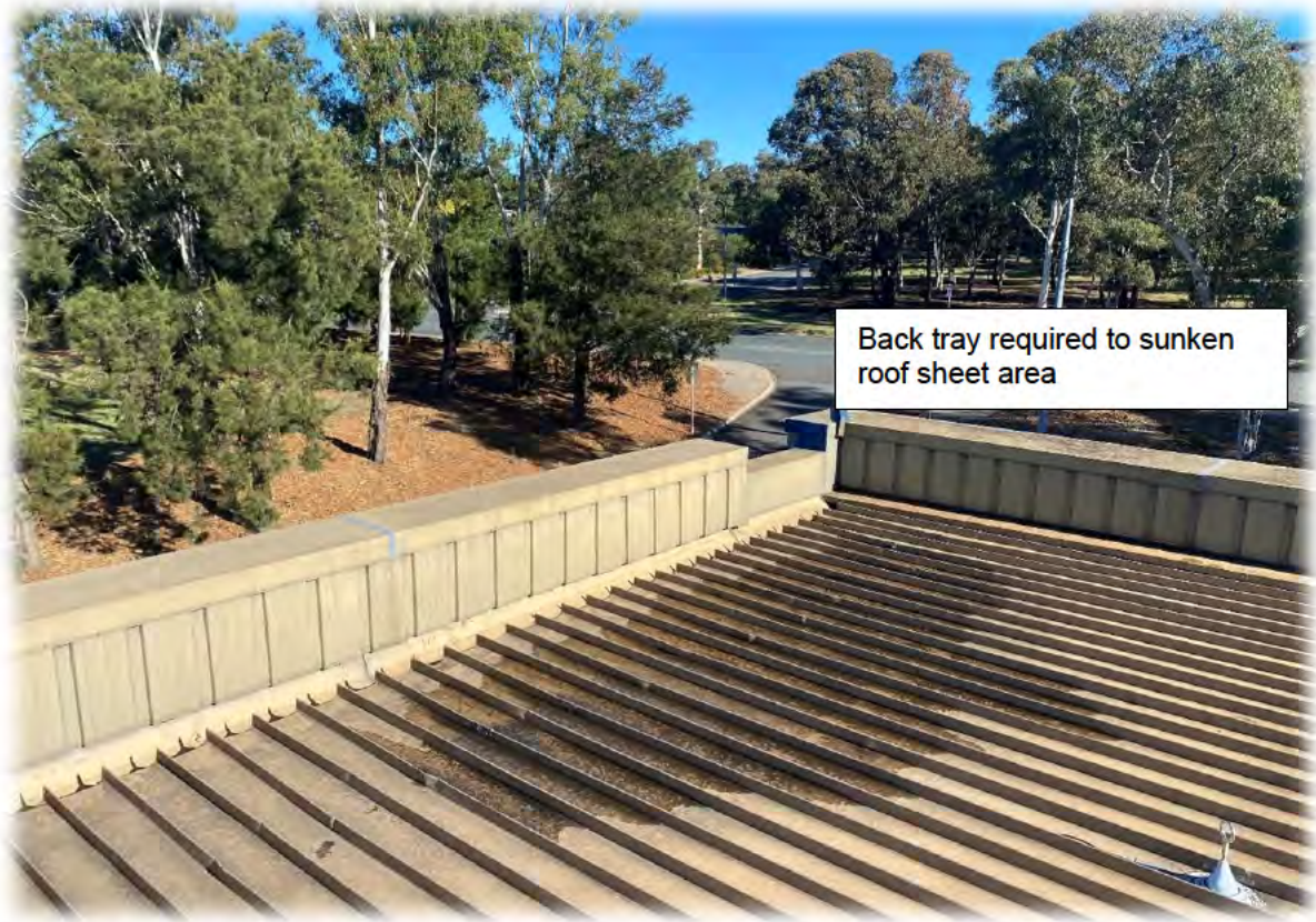
Figure 7: Pooling of water above gymnasium leak
