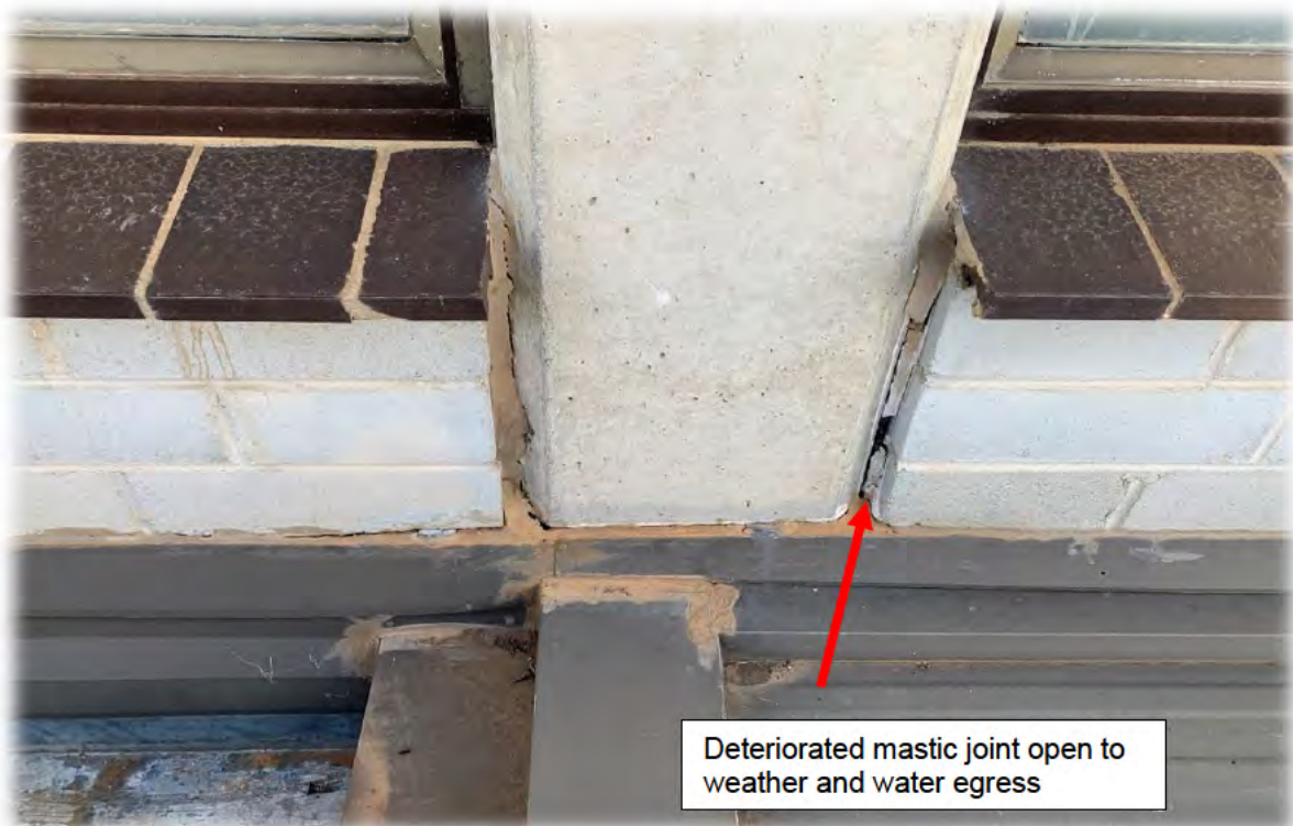
Figure 16: Deteriorated mastic seal along concrete wall joint
