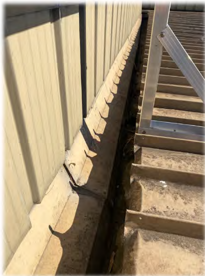
Figure 6: Gymnasium roof and perimeter box gutter showing loose and failed apron flashing
