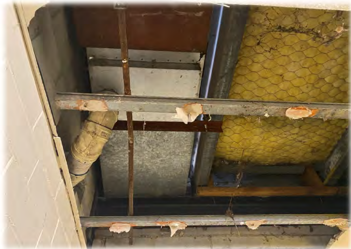
Figure 17: Ceiling leak in woodwork technology plant room
