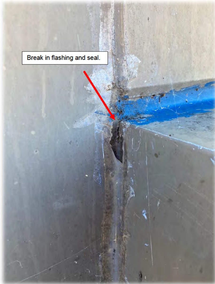
Figure 30: Break in flashing
