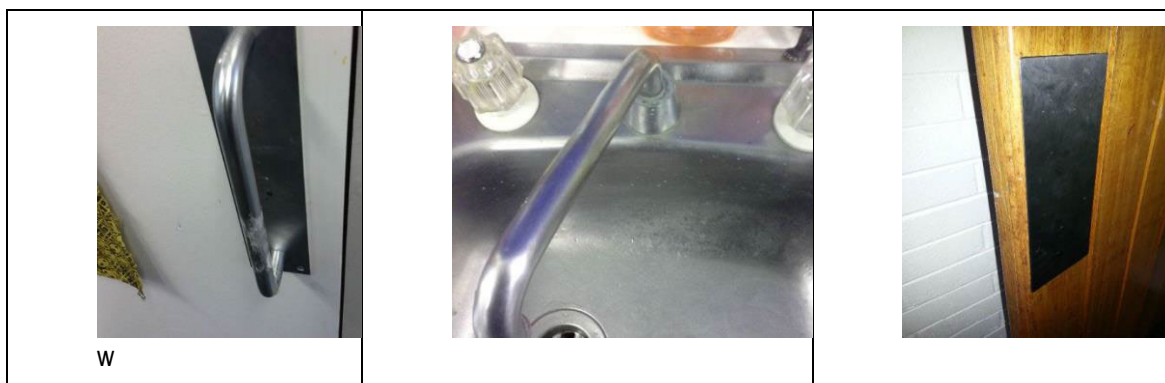
Figure 4: L -R Door Handle Hawker Primary; Sink - Caroline Chisholm; Door Push-plate Lyons Early Childhood school
