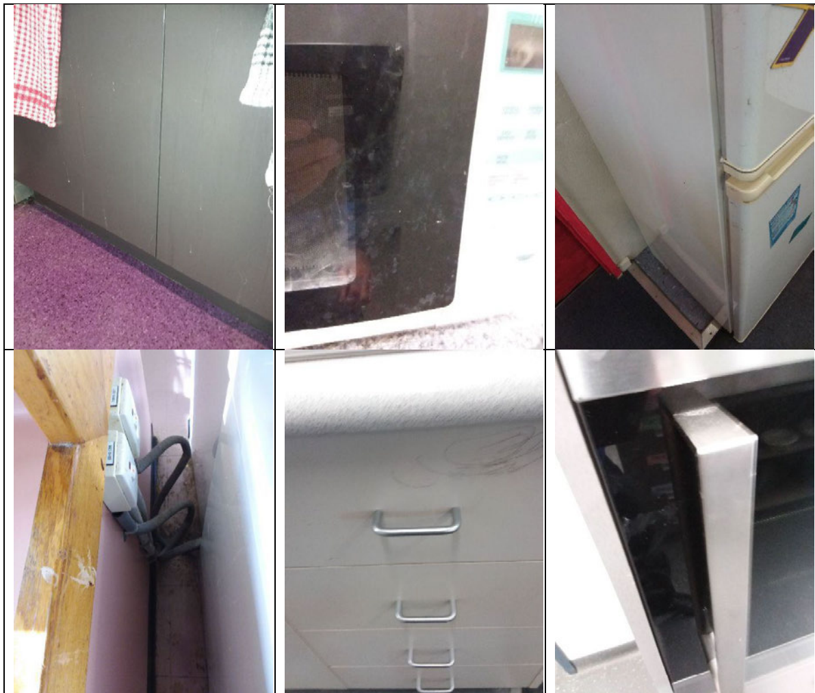
Figure 21: L-R Top: Kitchen Cupboards Harrison High; Microwave in cooking classroom Gold Creek Senior; Staff fridge Alfred Deakin High; Bottom L-R: Dirt and food residues between stove and cupboards cooking Classroom; Staff Kitchen Gold Creek high; Microwave Cooking Classroom
