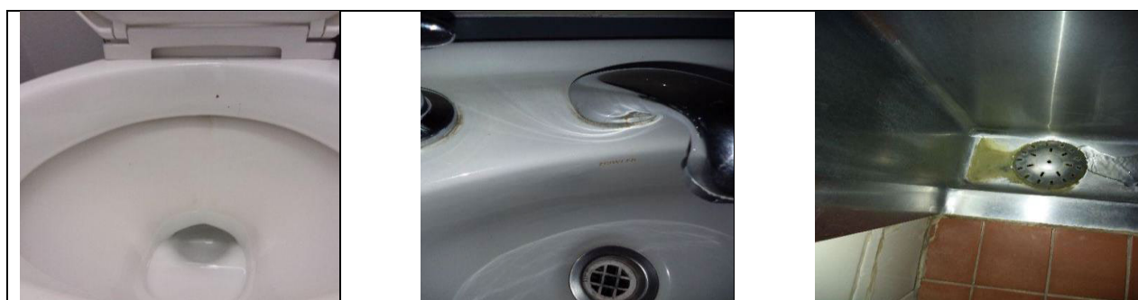
Figure 8: L-R: Faecal residue on toilet rim Gowrie Pre-school; Build-up on base of taps and sink drain & Urinal Palmerston North Primary
