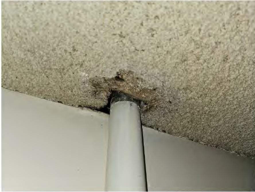
Photograph 1 Damage to exposed spray coating in the staff room
