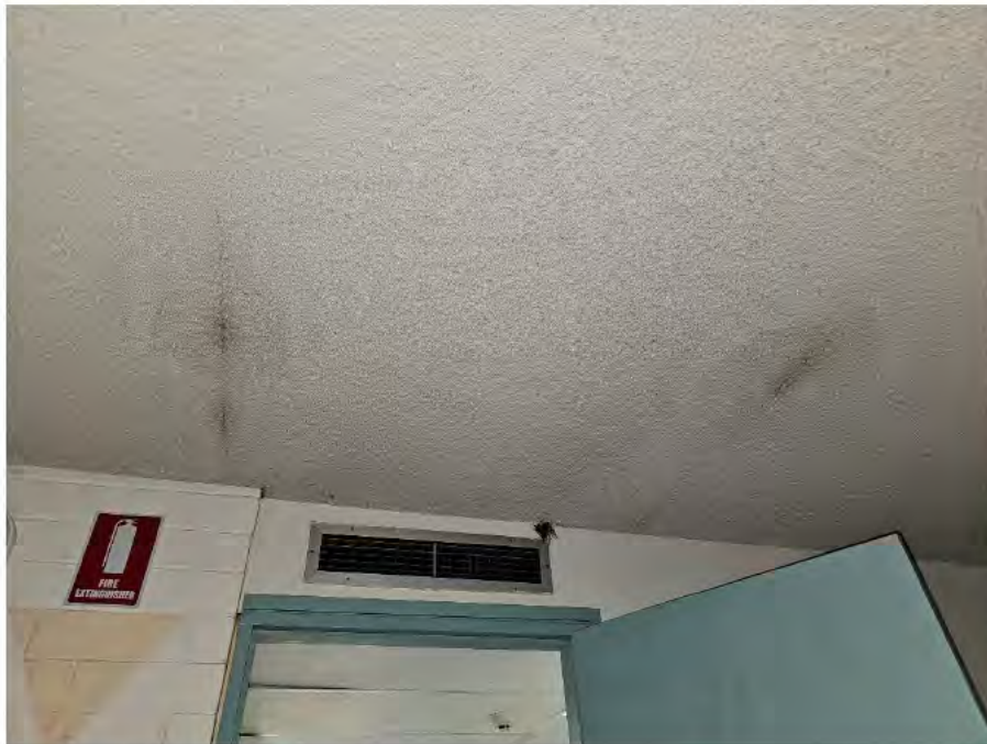
Photograph 2 Water damage to exposed spray coating in the staff room
