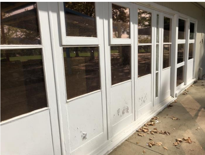
Figure 15: Pb13 Before Stabilisation 23/04/2019
