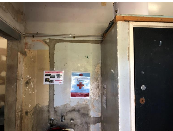
Figure 3: Pb03 Before Stabilisation 23/04/2019
