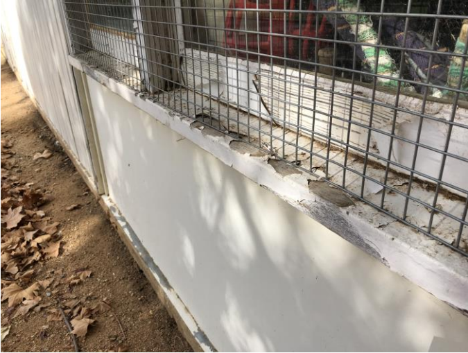
Figure 13: Pb12 Before Stabilisation 23/04/2019
