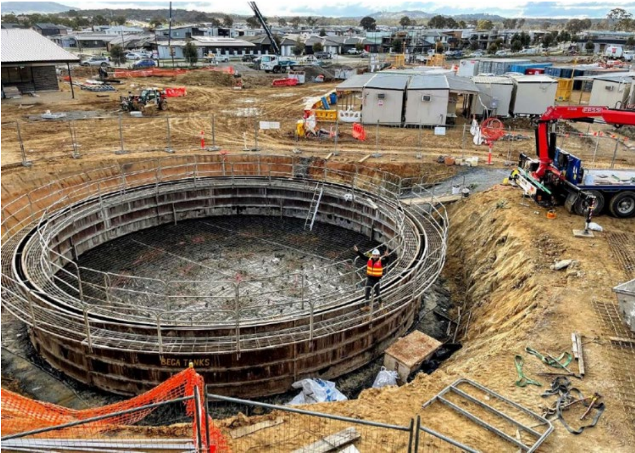
A 220 kilolitre inground water storage tank being installed at the new preschool to year 6 school in Throsby. The water harvested will reduce potable water use and keep landscapes and playing fields in good condition.
