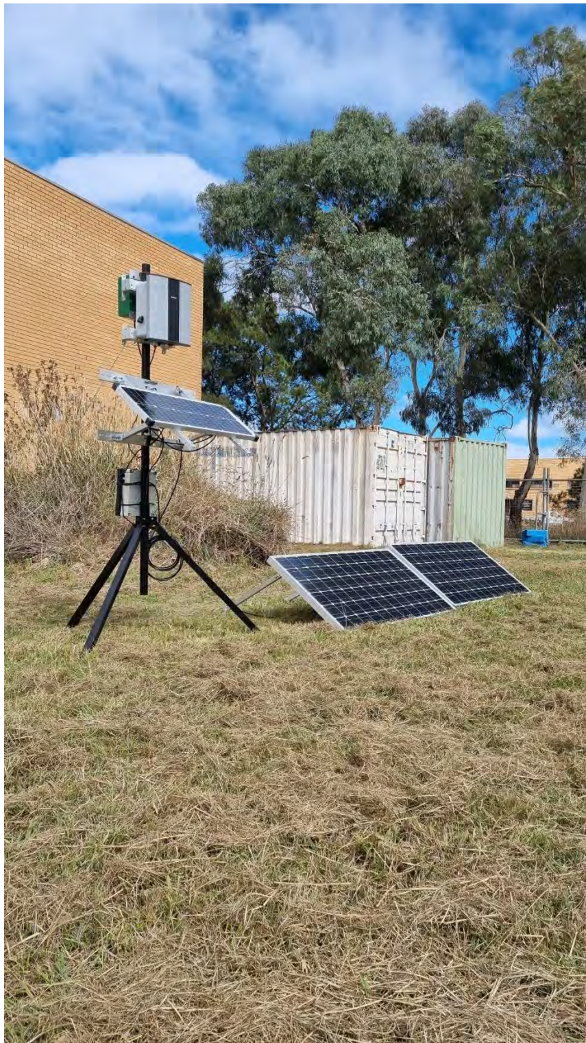
Figure B.2 Monitoring equipment installed onsite
